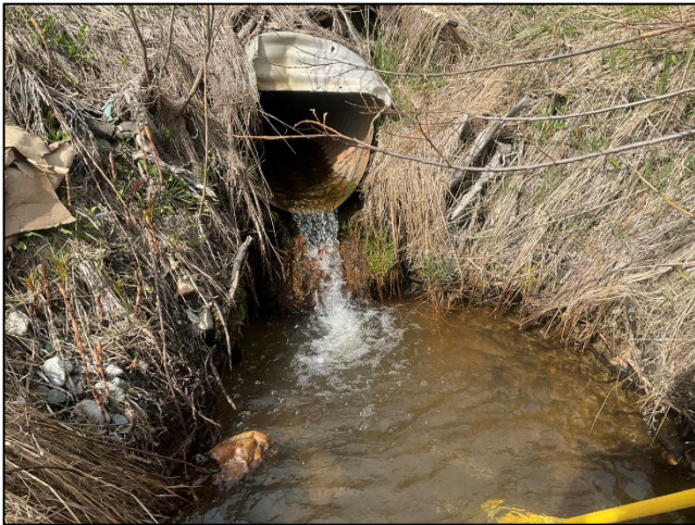
Figure 2.—Perched culvert at waypoint 1425.
